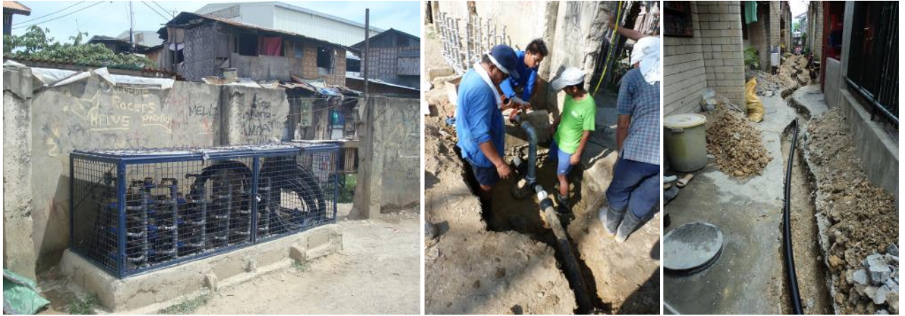
Lower Tipolo (Cebu, Philippines): Cluster – Connection to the bulk meter – Pipeline serving the houses
