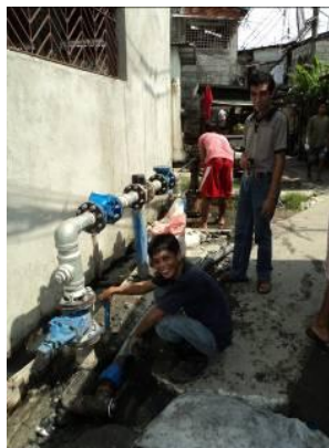
Cluster 1 connection to the bulk meter
